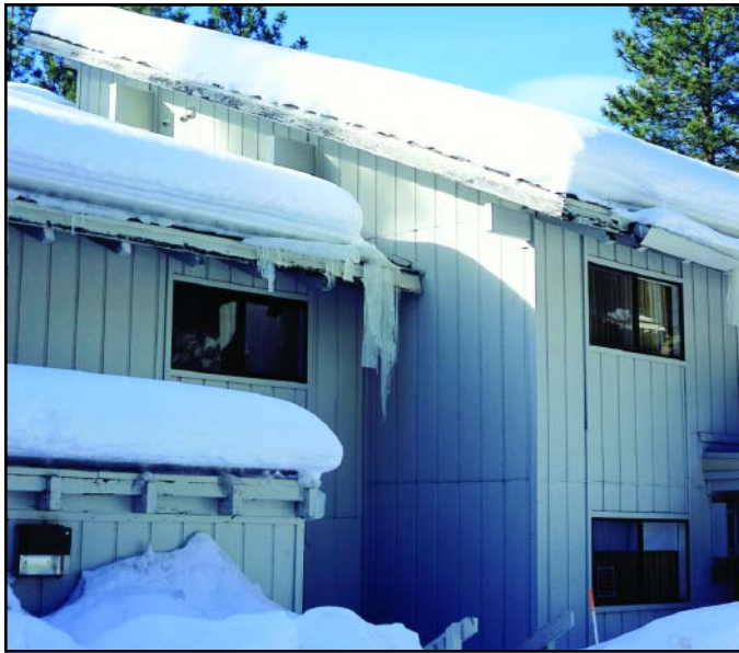
ROOFS IN THE LAKE TAHOE AREA MUST SUSTAIN HEAVY SNOW LOADS DURING THE WINTER MONTHS.
